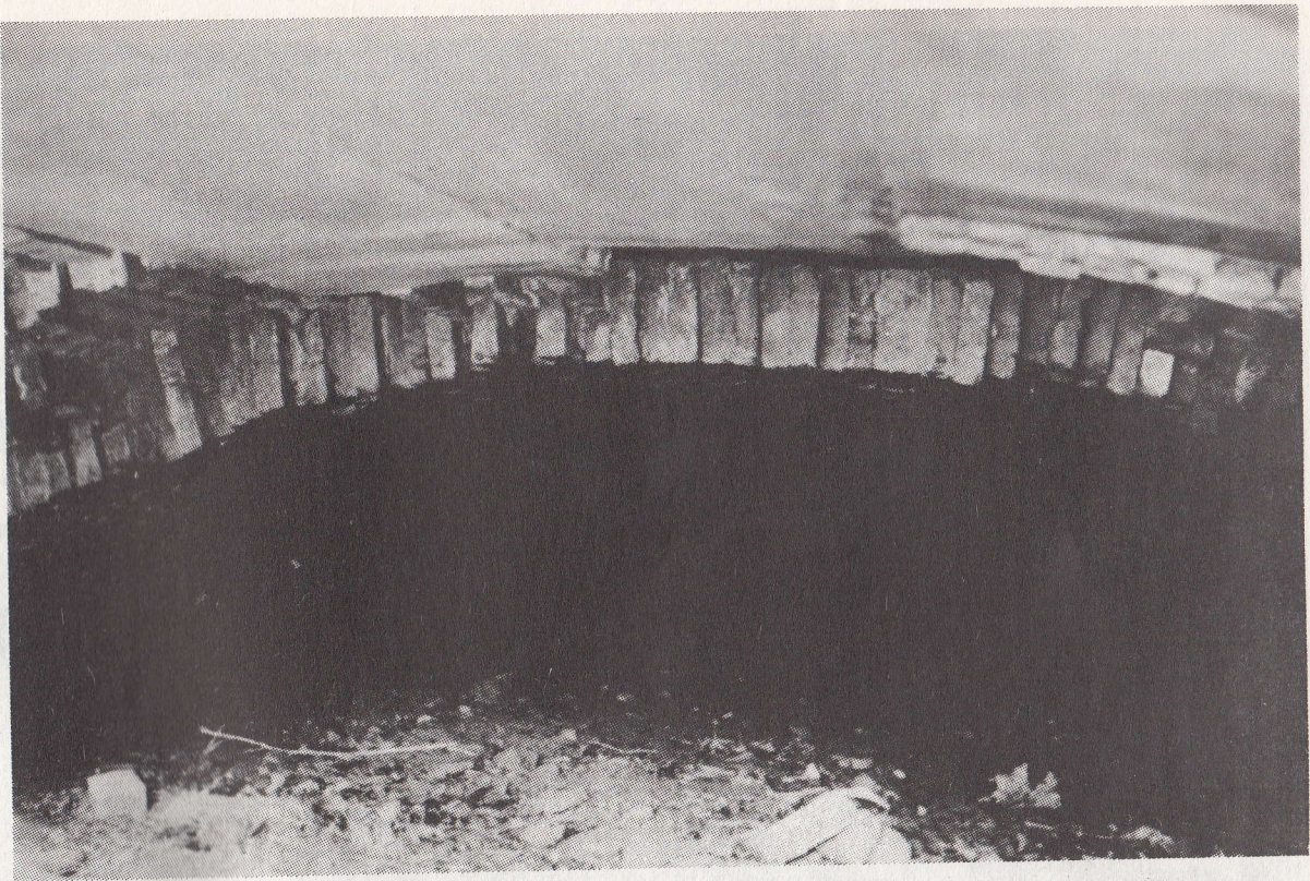
A look inside, showing the brick arch, which begins a few feet from the entrance, where the stonework of the Portal Facade ends.
