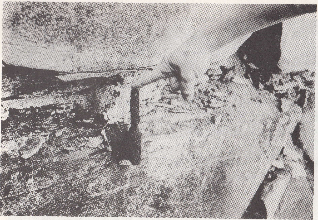
Hinge-pins for doors? Finger points out top of iron piece which has been leaded into the stonework. There are two of these on each side of the opening and others may be buried in silt.
