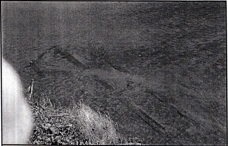
The Sugar Creek aqueduct foundation timbers are clearly visible in the water of the creek.
