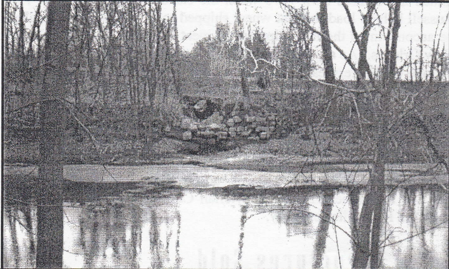
Top: Stones from the Raccoon Creek Aqueduct now surround a metal culvert on the south side of the creek. Photo by Bob Schmidt
