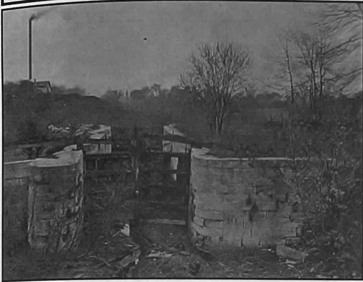
Locks in old discarded Miami & Erie Canal at Tipp City, Ohio Taken in 1924. Canal abandoned in 1913. From Neil Sowards
