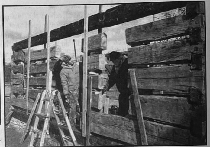
The logs were cut with chain saws to make door and window openings.
