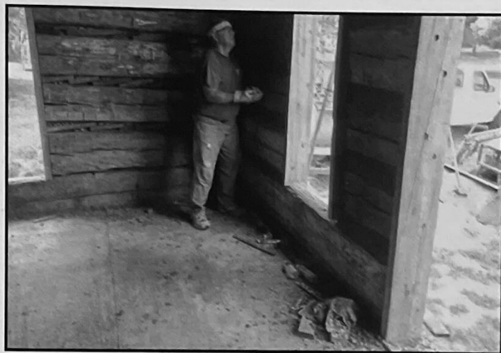
Placing "gob" (mortar) in the large cracks between logs was one of the jobs for the MWF crew. Here Dave Smith is busy inside covering the blocks of wood stuck between the logs. Then the interior was "whitewashed" to make walls lighter/brighter.
