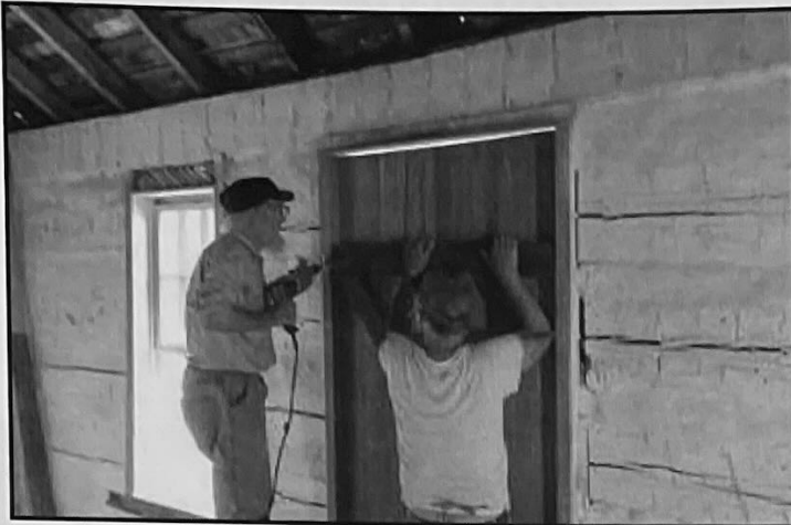
Roy Patrick and Brice Crowel hung a heavy rough cut wooden door on the entrance to the Loom House.
