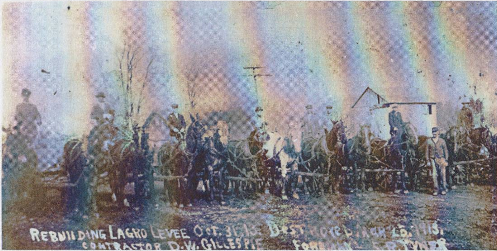
Rebuilding Lagro levee dated October 31, 1913. Contractor D.W. Gillespie and foreman S.R. Tyner are shown with their work gang. Photo by E.S. Shelton. Courtesy of Today's Catholic , Diocese of Fort Wayne-South Bend.
