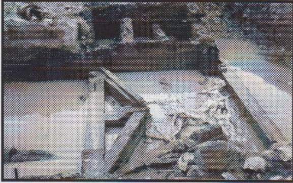
Some of the most impressive pieces of the lock were those that formed the mitre sill upon which the west gate closed. Photo by Bob Schmidt
