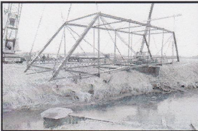
The Stearns Truss Bridge was removed by cranes from its place over Big Monon Ditch and is being rehabilitated. Photo by Dan McCain
