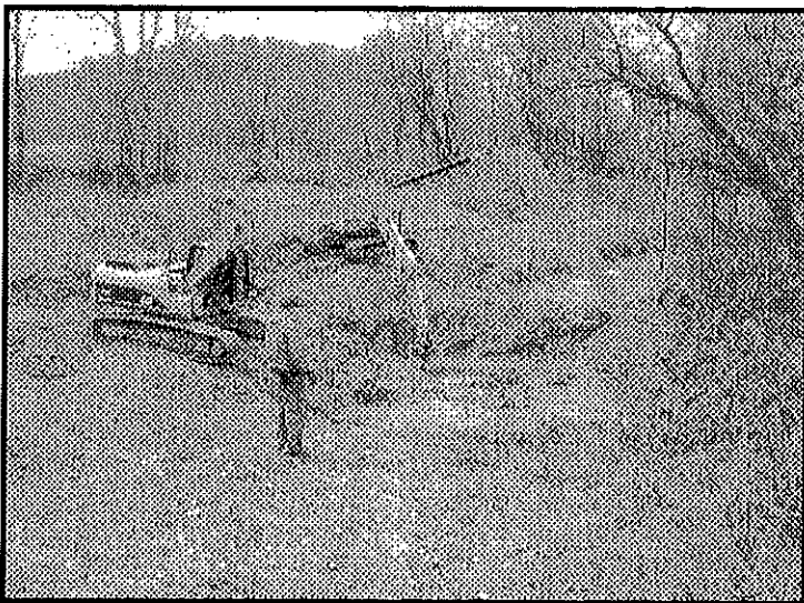
The Feeder Dam across the west fork of the Whitewater River for the Whitewater Canal underwent repair the past year.
