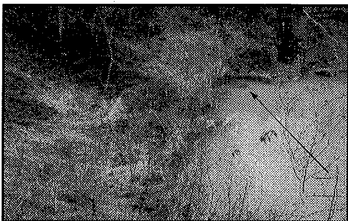
Only the top of the Big Tunnel is visible. Photo by Bob Schmidt
