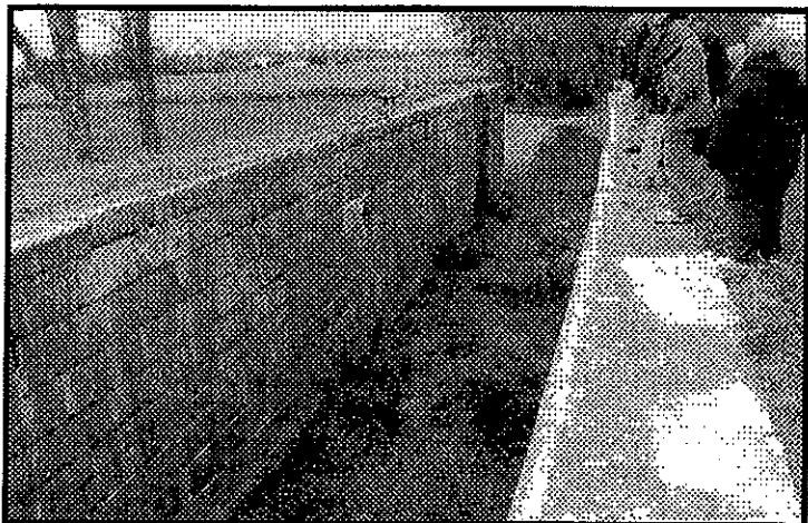
Lock 8n's walls are very straight. Its capstones are in tact. The farmer keeps the land around it nicely mowed. The gate recess is visible. The tumble is located to the right and is not seen.
