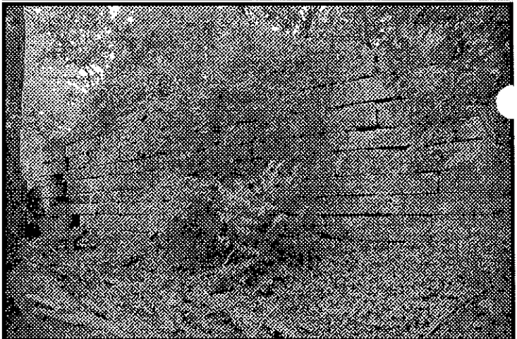
Above: Remains of towpath/buggy bridge at Wild Cat creek Photo by Lynette Kross
