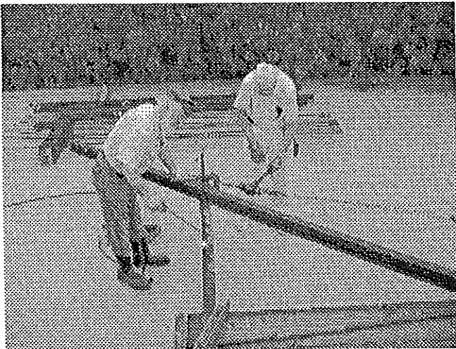
Beginning the heating process while Ron "feels" the pull on the winch
