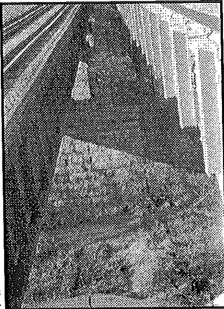
Abutments of Dry Fork Aqueduct remain between railroad and road bridge over Dry Fork Creek. Photo by Bob Mueller
