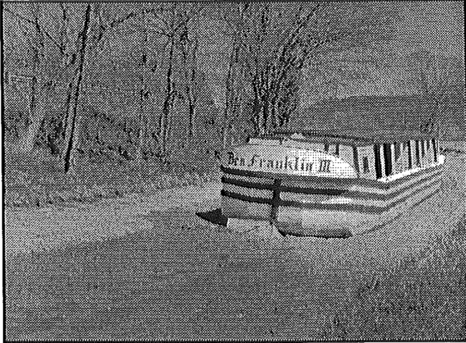
The Ben Franklin III rests in the dry Whitewater Canal bed in Metamora while a lock and aqueduct repair project and dredging are underway. Photo by John Bower —Studio Indiana
