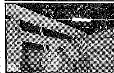
Top: Ed Gruber and Roy Patrick worked outdoors fitting the mortise joint into part of the miter edge that touches the second gate when both are closed.
