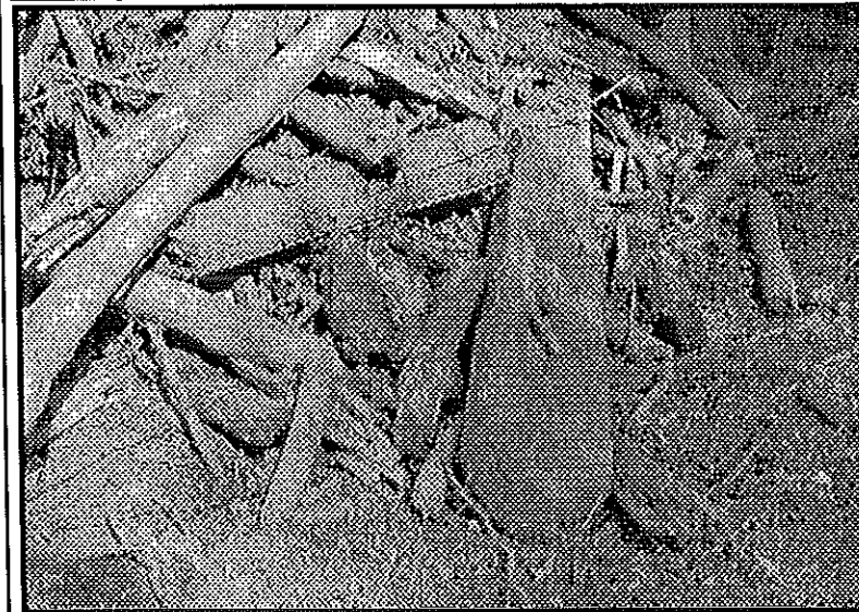
Prairie Creek Arch in Miami County has deteriorated over time. These pictures show its condition and the timbers that were recently removed.
