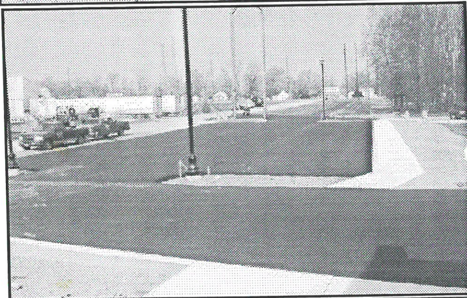
The black top drive and parking lots for the Canal Conference and Interpretive Center in Delphi, IN are finished and the building nears completion. Photos courtesy of Dan McCain
