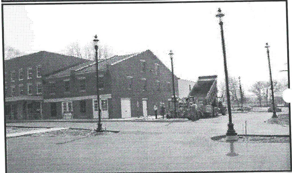
Top: The trail overlooking the Wabash River was completed using the weighting material for the Center's foundation. Photos courtesy of Dan McCain Bottom: Delphi's beautiful new CANAL CONFERENCE & INTERPRETIVE CENTER is progressing nicely. The blacktop drive and parking lots are down. Final outside grading was completed so that Canal Association's volunteers could landscape on May 17th. Logansport contractor Leo Brown Construction should complete the last of the 12,000 square foot $2 million dollar building by the end of May. Painting and carpeting are done. Finishing and installing exhibits in the museum area remain to be done and need further funding. Your extra dollars would be greatly appreciated. Mail to: Dan McCain, Carroll County Wabash & Erie Canal, Inc., 3198 N 700 W, Delphi, IN 46923-8261
