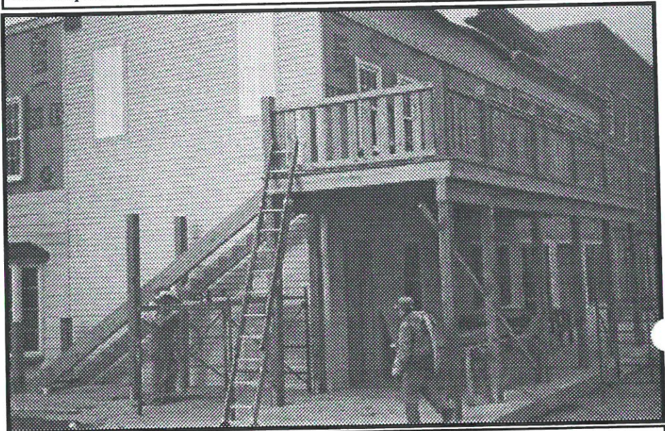
The facade of the Buford House nears completion on one end of the Canal Conference and Interpretive Center being built in Delphi, IN. Photo by Dan McCain
