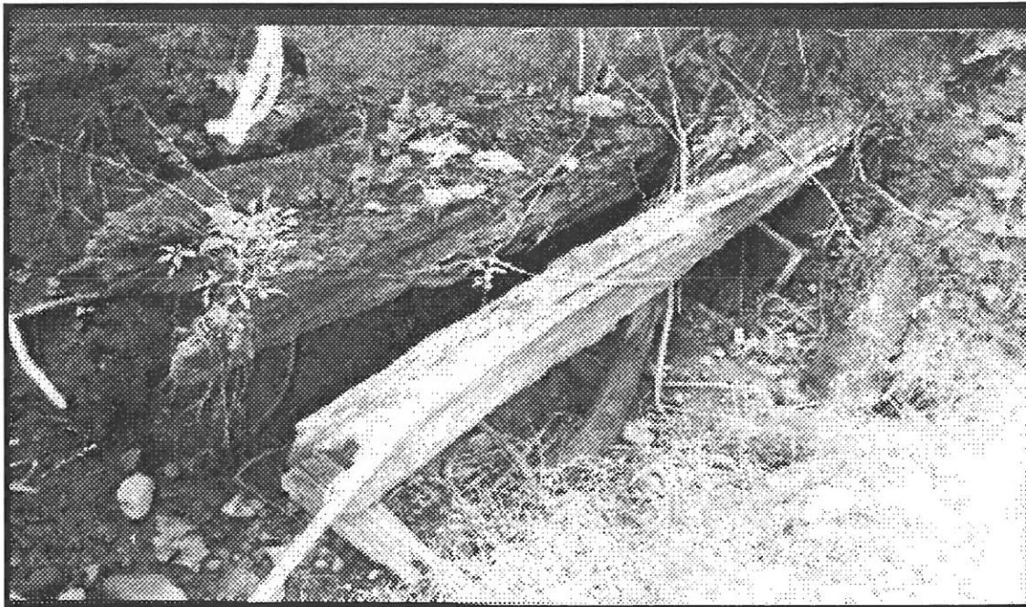
Timbers of Culvert 52 of the Wabash & Erie Canal in Wabash county, IN were discovered by Charlie White. This photo was taken looking toward the south and is of the east span of the culvert. Photo by Tom Castaldi
