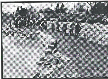
The Maumee River was high so that only the top of the arch culvert could be seen. The new concrete retaining wall is made to look like stone. Photo by Dr. Tom Grimes
