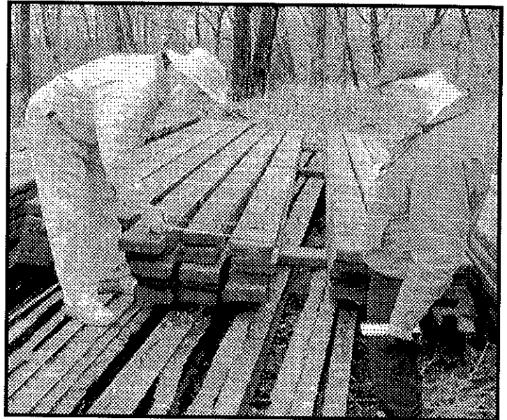
MWF volunteers decided we needed all the salvaged materials from the bridge. The old flooring and 'I beam' floor stringers were mostly still good. They will be delivered to Canal Park as part of an agreement with Putnam County Commissioners, INDOT and the Canal Association.
