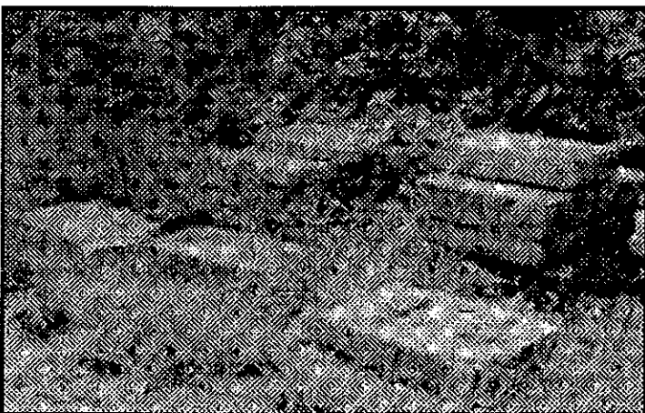
Above: Locally quarried stone will be used at the lock site for steps from (6) to (7) and the "landing" at (7). Top Right: Trail path has been graded along railroad embankment from (1) to (2).
