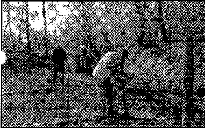
Volunteers build fence along field (3) to (5) to keep visitors on Whitewater Canal Trail easement.
