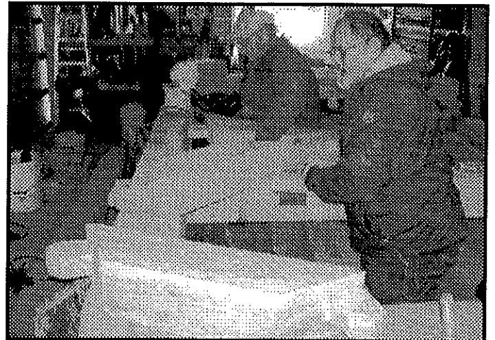
Brice Crowel and Ron Scowden make cuts to fit the braces to the beams. This pre-fab operation is done inside this winter. Next Spring the beams will be up-righted at the scale site to support the roof.
