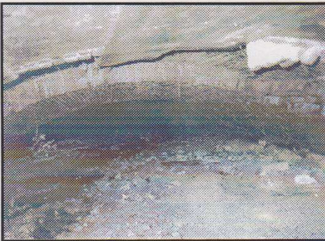
Looking Inside North Tunnel Portal Note Brick Ceiling and That The Tunnel Has Been Filled with Dirt and Rocks Photo - Brian Migliore
