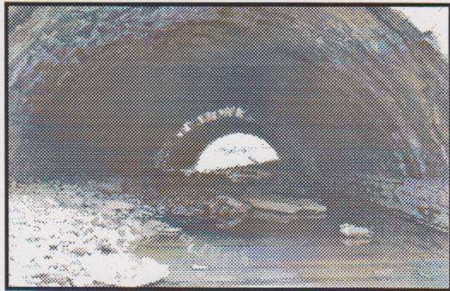
Butlers Run Culvert Brookville Note Light Shining Through Hole in Center of Culvert and 18 Inch Wide Timbers Supporting the Culvert Photo Brian Migliore
