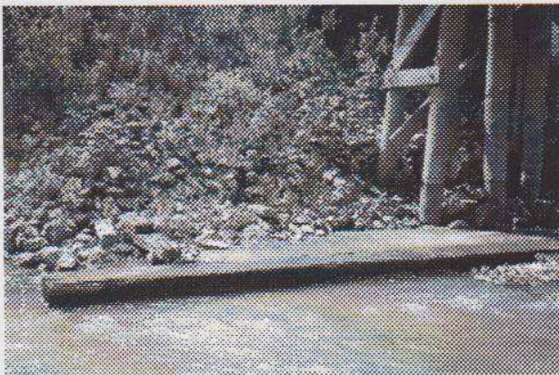
SEE REMAINING TIMBERS IN CREEK BED PHOTO - BOB SCHMIDT
