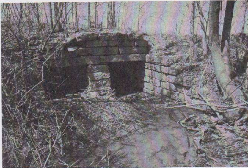
The only remaining double box culvert on the Extension is north of Ottoville, on CR25M at CR O.
