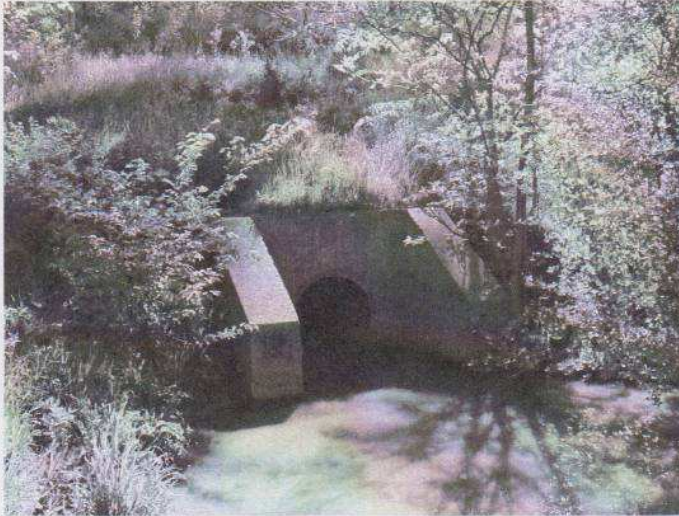
Staley's Culvert was south of Newberg and was a simple concrete tube with concrete wing walls.
