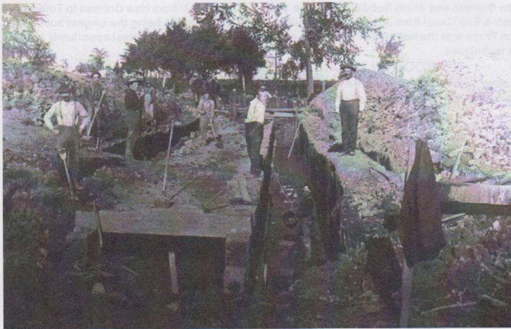
Wooden Culvert over 6 Mile Creek, north of Spencerville, being rebuilt. (Allen County Museum)
