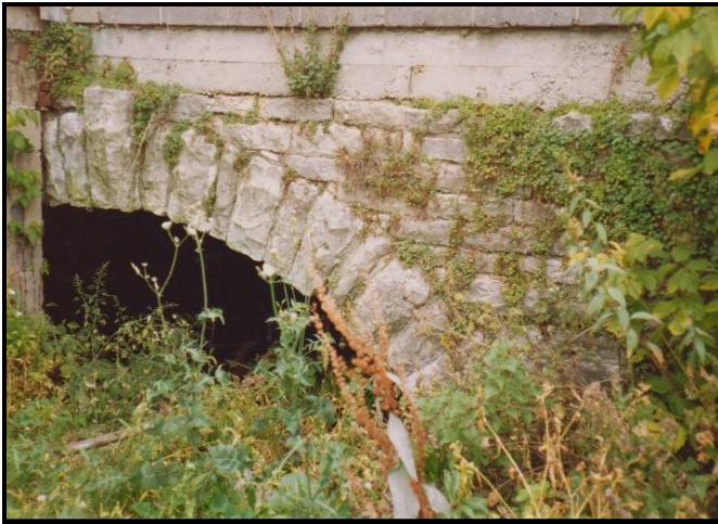
Today this culvert under the National Road that connected the Whitewater Canal on the south to the Hagerstown Extension on the north has been filled in by a wall of concrete blocks. Photo Bob Schmidt
