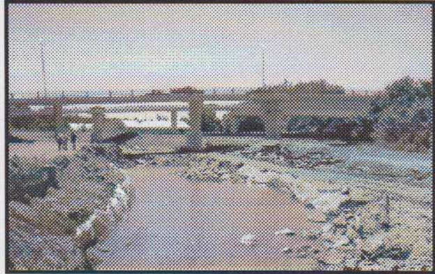
The timbers on both sides of the canal were covered with plastic to keep them from drying out. Photo by Bob Schmidt
