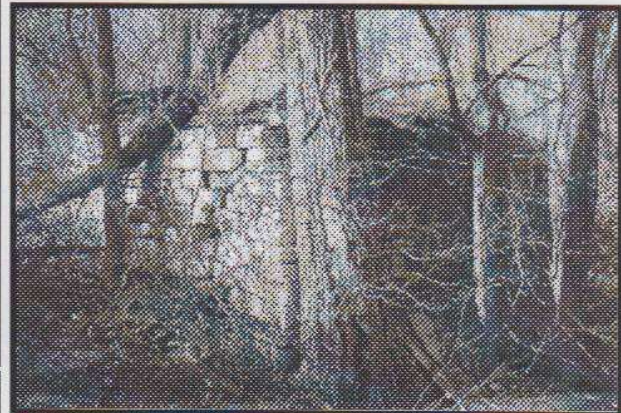
This abutment for the tow path bridge is on the west side of Wild Cat Creek. Photo by Bob Schmidt
