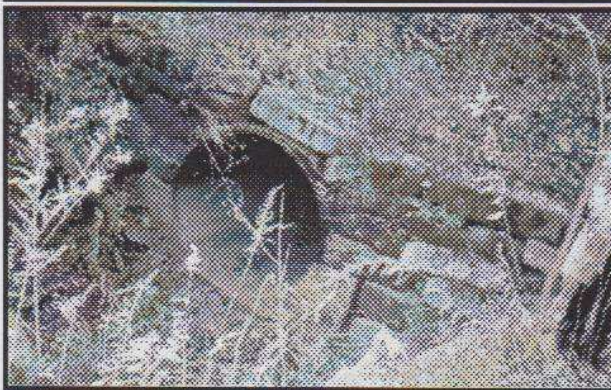
This drainage culvert is where Aqueduct #12 crossed Big Raccoon Creek. Some of the stones from its was used around the culvert. Photo by Bob Schmidt
